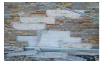
Delamination of Stone
